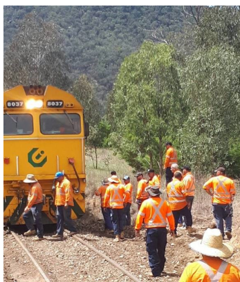
DOWN THE TRACK: Work on re-opening the rail line has been underway since late 2017
