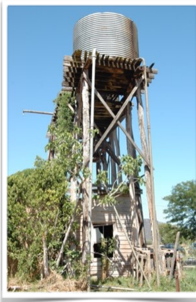
Water tanks on 'Tarwyn Park'. ©S. & M Andrews
